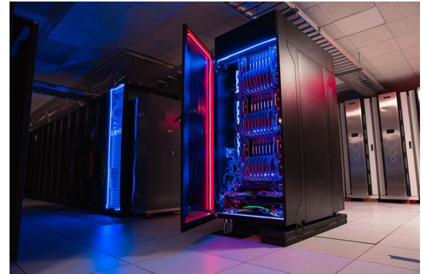
Cosmos in SDSC data center
