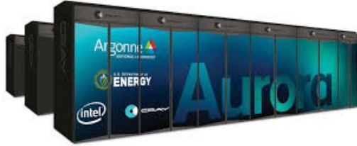
Intel CPU + GPU Based (Recently installed)
